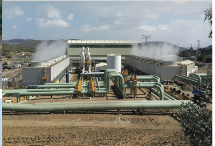
Geothermal plant in Naivasha; Ksh 8.6bn for Geothermal development
